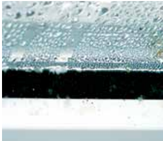
Higher risk of condensation and mould formation due to conventional aluminium spacers
